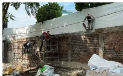
Before Rectification Works
